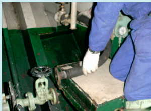
Illegal pipe – sludge pump to overboard
