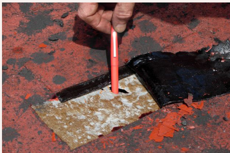
A hole in a main deck – found masked with tape painted red
