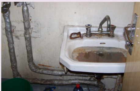
Sanitary facilities not fit for use
