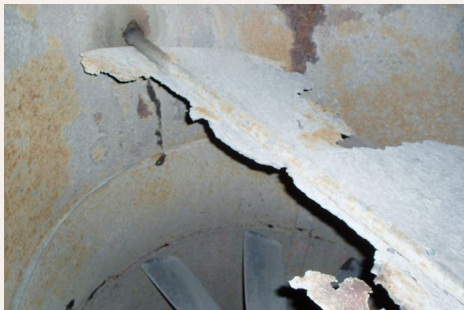
A wasted engine room fire damper
